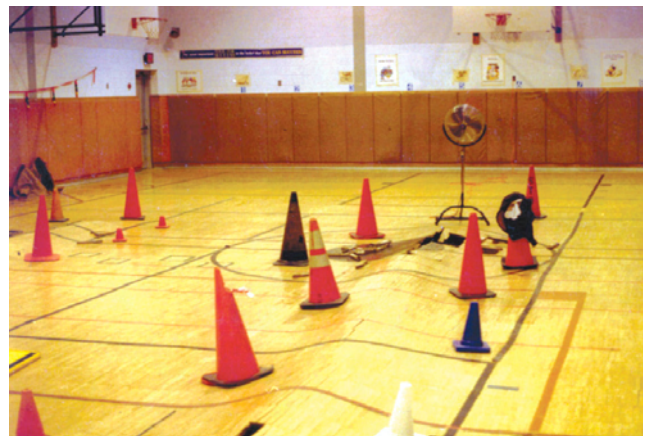
Photograph 2: Buckling Wood Floor —If wood is not conditioned to the mid point of its expected moisture content range prior to installation it will buckle.
