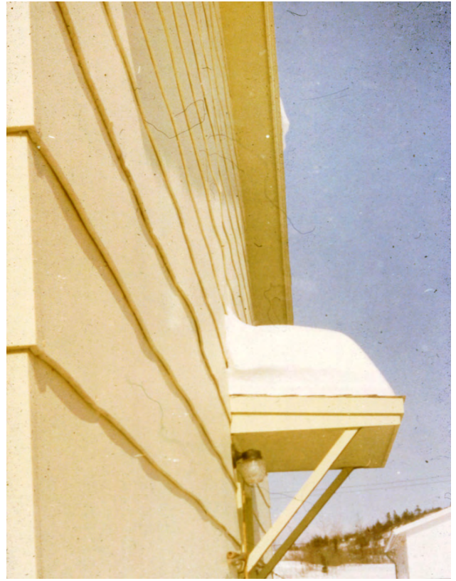
Photograph 1: Buckling of Hardboard Siding —Hardboard grows along its length as relative humidity (and therefore moisture content) goes up. Since it is nailed every 16 inches its movement along its length is restrained and therefore it buckles.
