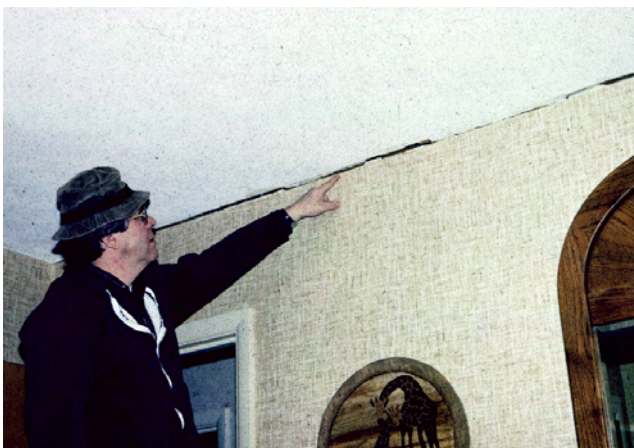
Photograph 4: Truss Uplift —Gypsum board ceiling cracks at interior wall ceiling connections due to truss uplift. Trusses move up in the winter and come down in the spring. Ah, the changing of the seasons, leaves change color and fall, and the trusses move up while the birds fly south.
