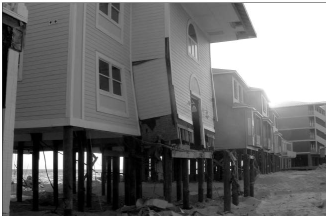
Figure 1. Stairs did not break away cleanly, resulting in damage to the elevated building.
