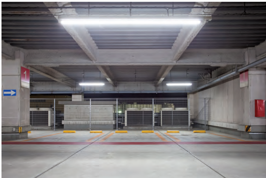
Public garage ventilation system
