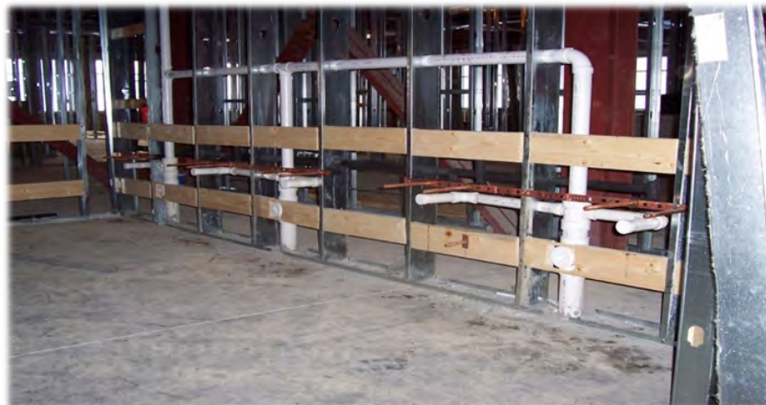
Photo of a typical multiple lavatory rough-in
