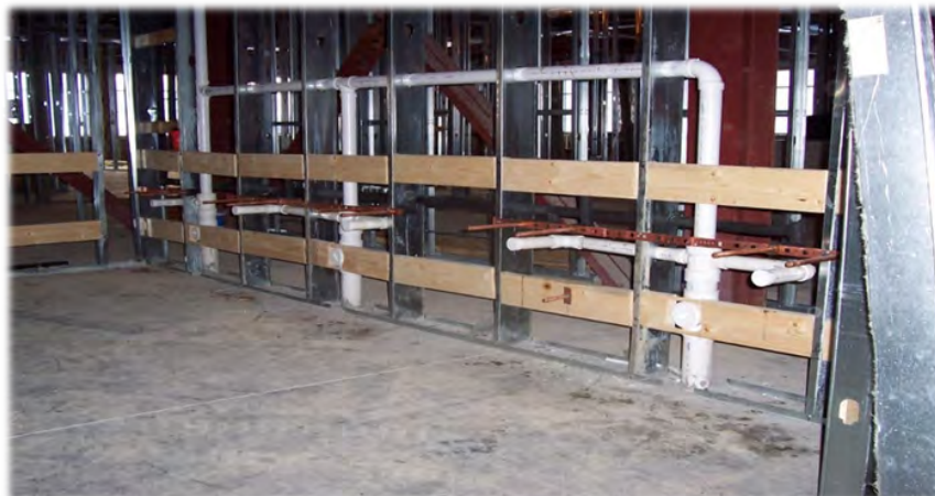
Photo of a typical multiple lavatory rough-in
