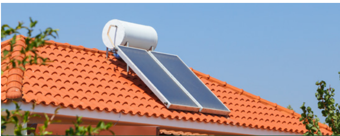
Figure 4. Roof-mounted thermosiphon solar water heating system
