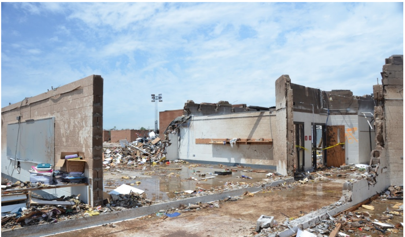
Figure 1. Damage to the New Main Classroom Building at Plaza Towers Elementary School. The seven schoolchildren died in the central hallway when the classroom walls collapsed on them. An additional two staff members and one student were injured in this building.
