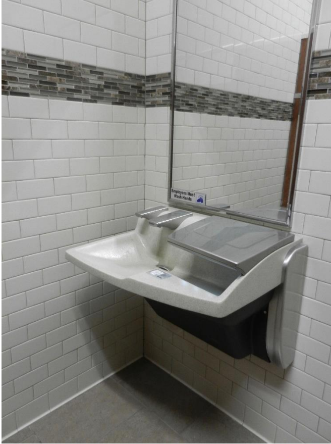
Hand dryer in the lavatory.
