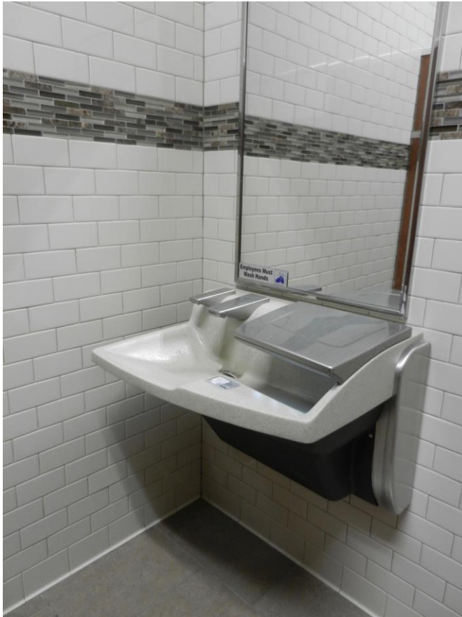
Hand dryer in the lavatory.
