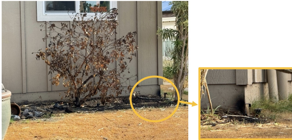
Figure 1. 6-in noncombustible vertical clearance worked as fuel break at the base of exterior walls in Lahaina wildfire. Photo credit: Steve Hawks, IBHS.
