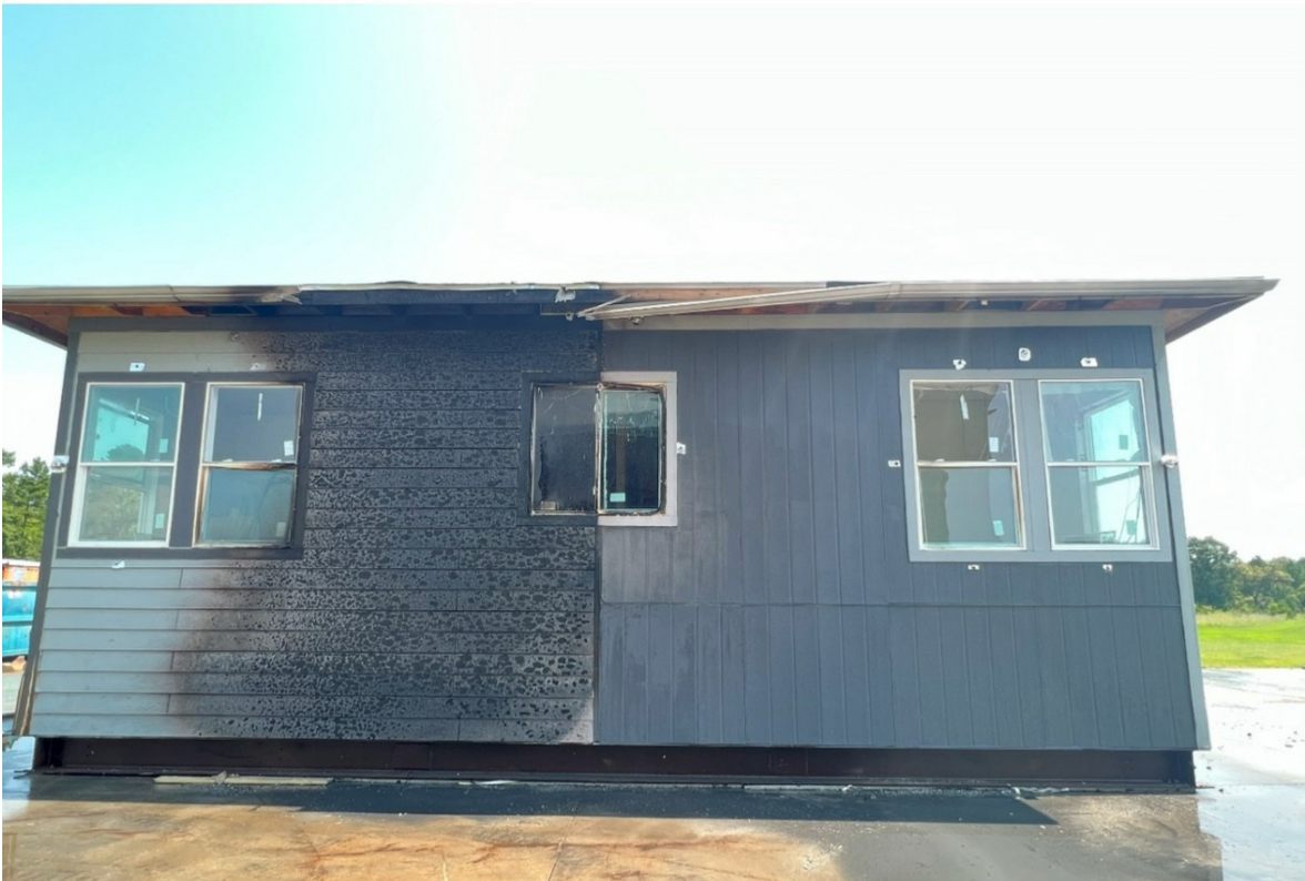
Figure 1. d. after suppression; severe damage can be seen on all components on the left-side.
