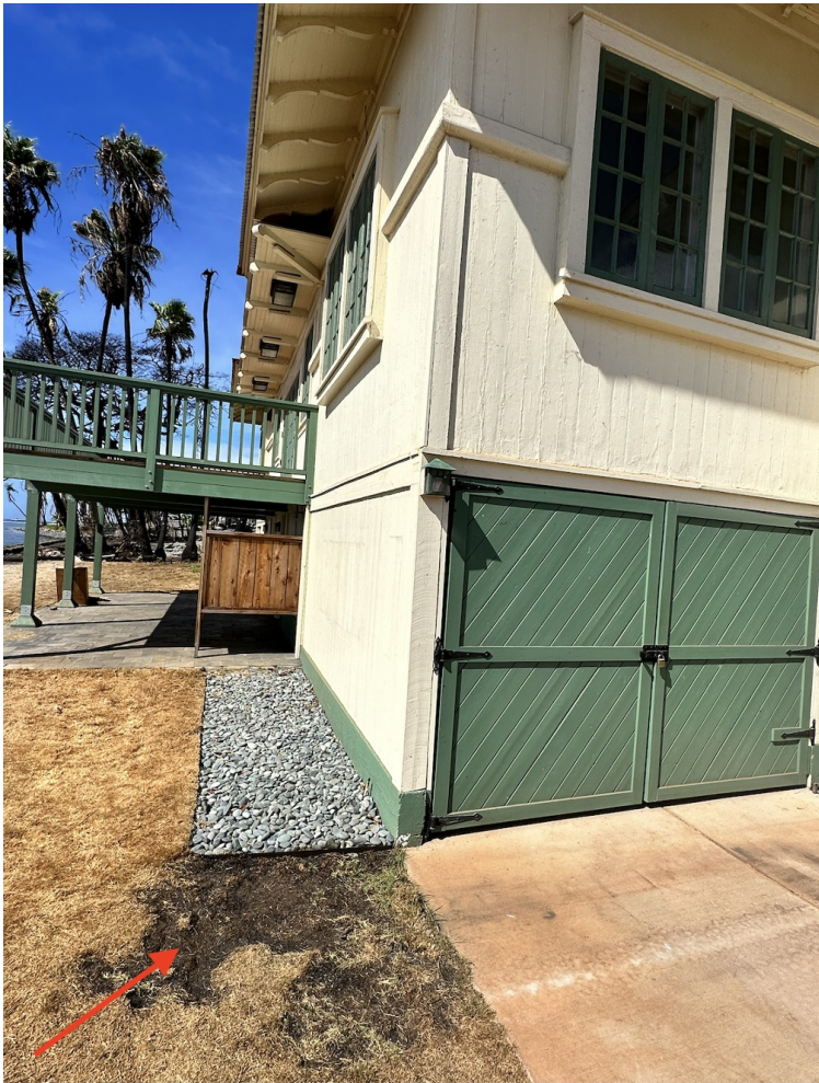
Figure 2. Noncombustible mulch breaks the fuel path in Lahaina wildfire. Photo courtesy Milad Shabanian, IBHS.
