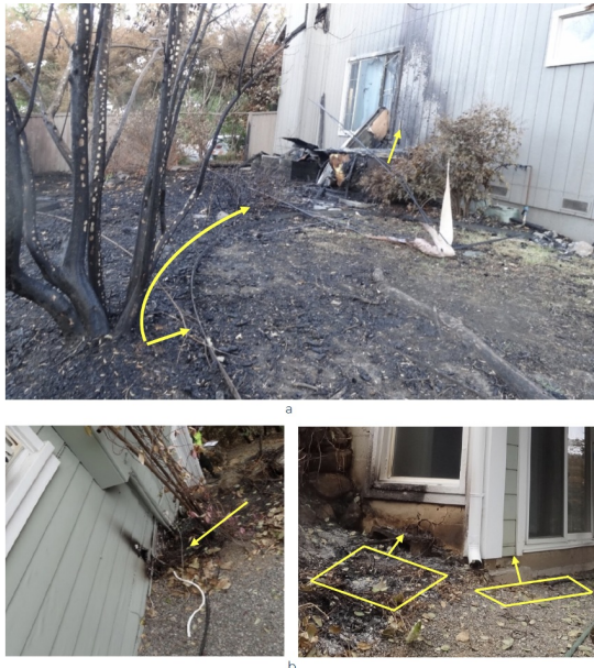
Figure 1. Example of vegetation in small amounts located in Zone 0 creating a pathway for fire spread: (a) Wood mulch provided a pathway for fire to get close to the building and ignite a hot tub during the Glass Fire (2020) in Napa and Sonoma Counties, California; (b) Ground-level plants during the Glass Fire (2020).
