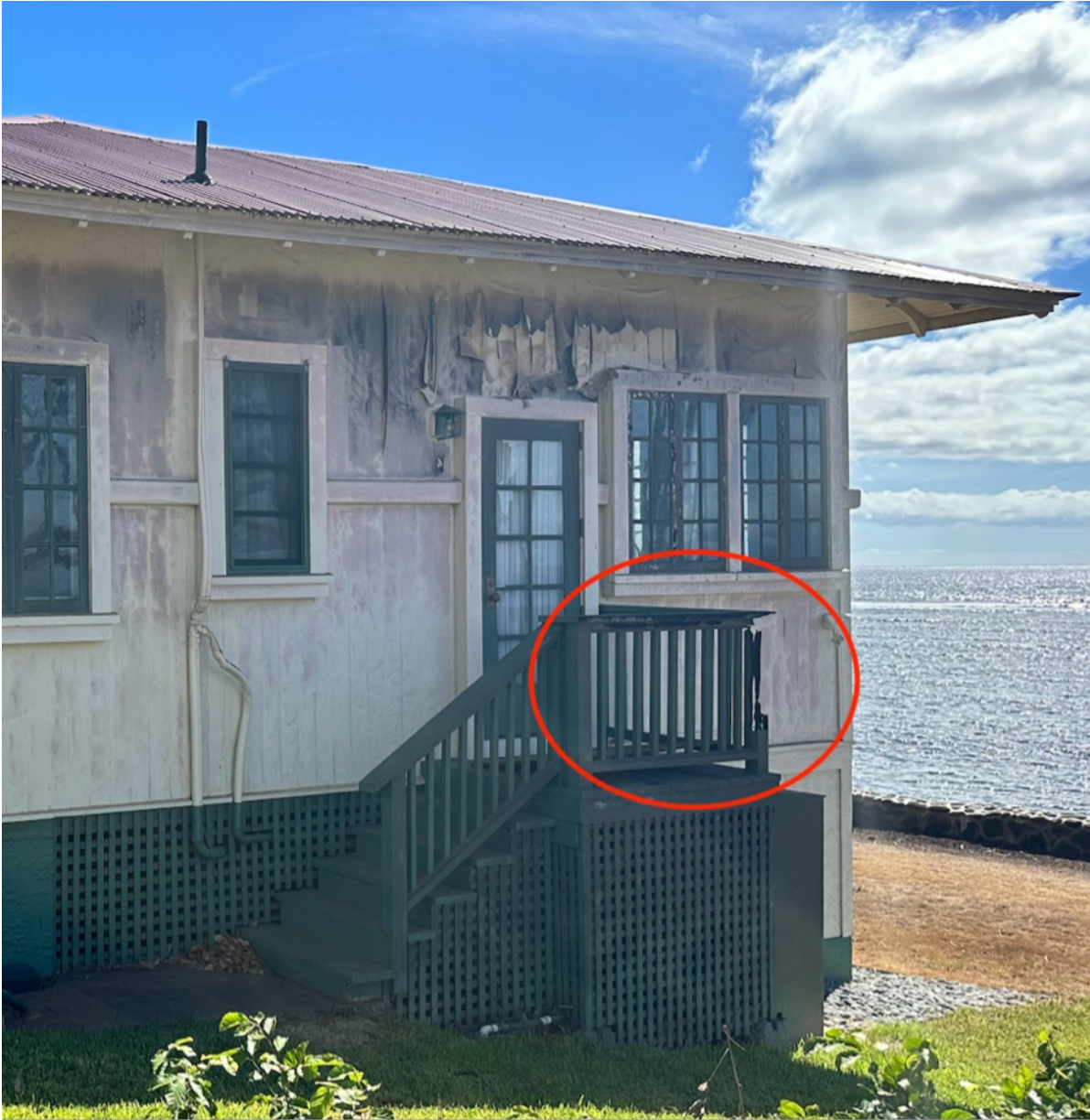
Figure 1. Nonconforming attached accessory structure (stair). Photo by Milad Shabaniyan, IBHS.
