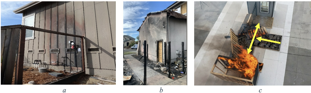
Figure 1. Examples of combustible fencing providing a pathway for fire to the house, damaging the noncombustible siding.
