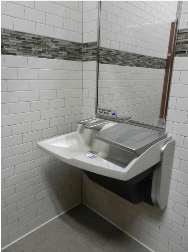
Hand dryer in the lavatory.
